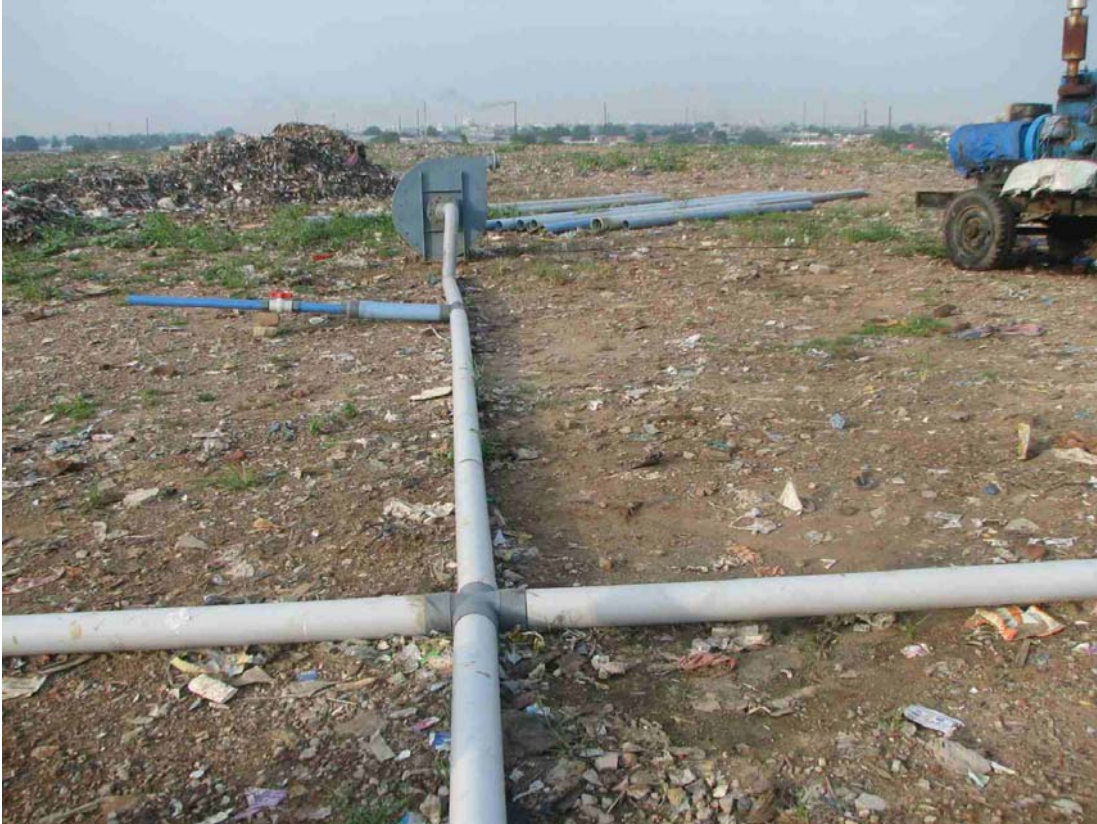
Figure 3-5. Pump Test Blower and Collection Piping
