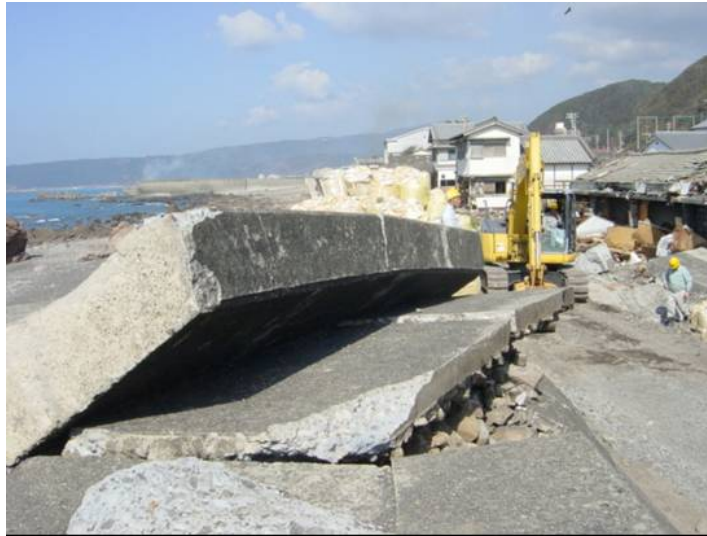
Figure 10 Photograph of the damage caused along the Nabae Coast in Kochi Prefecture Kochi Prefecture
