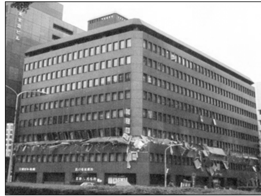
Fig. 4: Ten storey building with collapse of third storey
