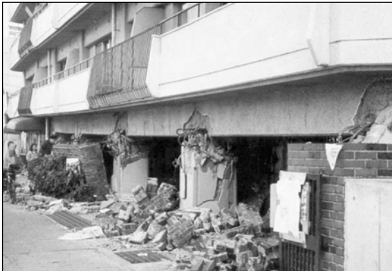
Fig.3: Soft ground storey failure
