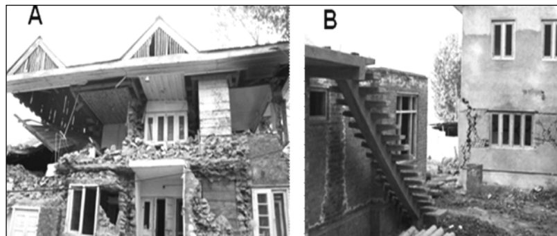
Variation in damages to buildings located in nearby areas shows that better quality of construction can perform much better during seismic event.
