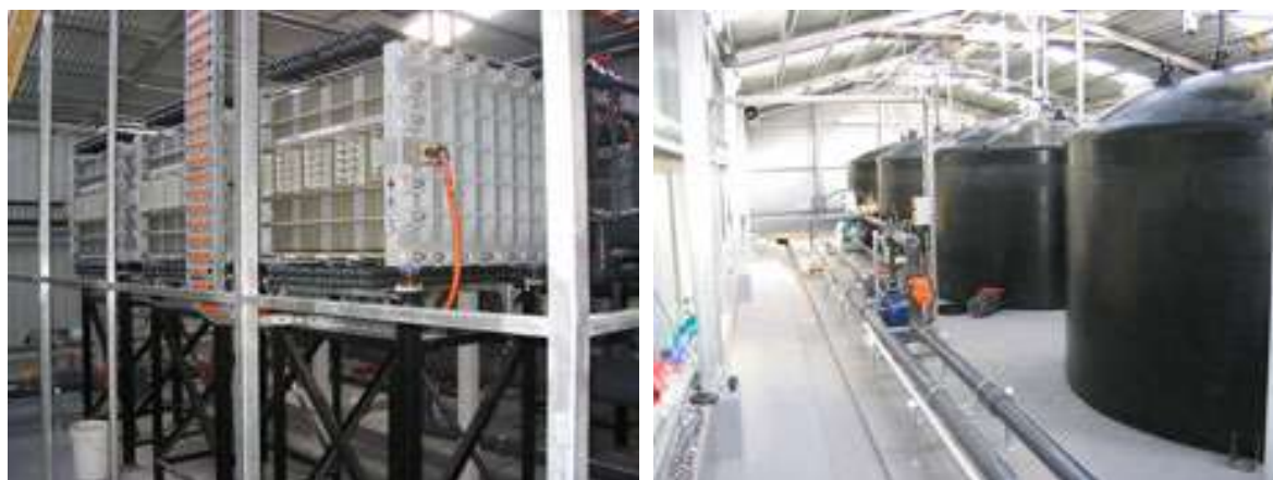
Figure A.19 (right): Electrolyte tanks
