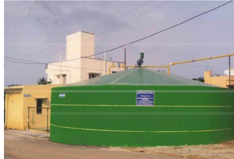
Bio-mechanization plant – 5 MTPD capacity each at 13 locations
