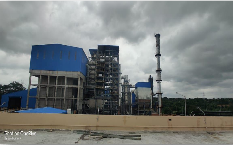
Waste to Energy Plant- BBMP
