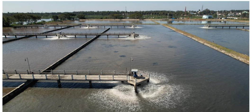
24.57 MLD Aerated Lagoon Type STP – Tumkuru CC, Tumkur Dt
