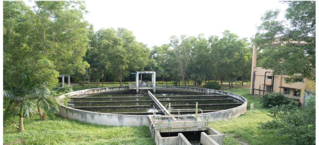
40 MLD SBR Type STP - HDMC CC, Dharwad Dt.
