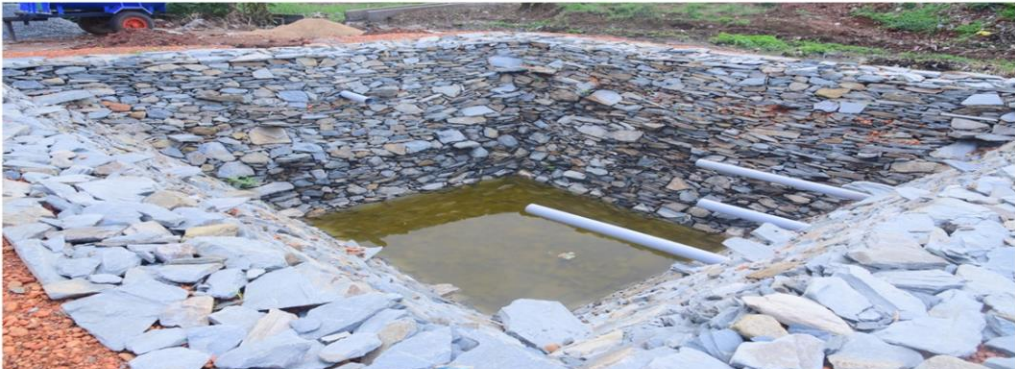
Waste Stabilization Pond at Kodyala GP, Haveri Dt.
