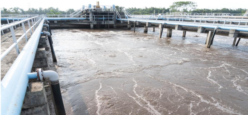
40 MLD SBR Type STP - HDMC CC, Dharwad Dt.
