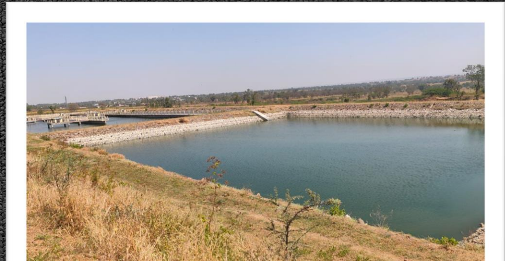
30 MLD Aerated Lagoon Type STP – Bellary CC, Bellary Dt.
